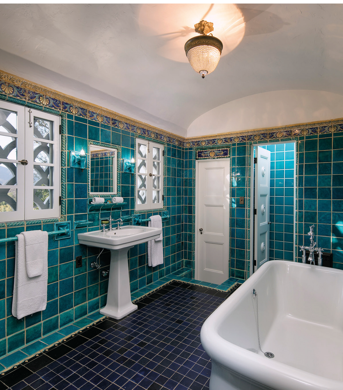
A tile doctor ensured damage to the original art deco tile throughout the home was kept to a minimum when installing updated plumbing fixtures. One would never think the master bathroom's new shower and water closet weren't original.
